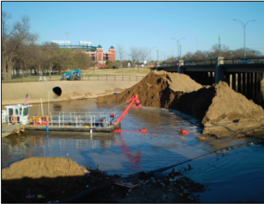
With Ranger Stadium in the background, the dredge chips away at the stockpiled material in the creek and pumps it 1.5 miles to a settling basin.
